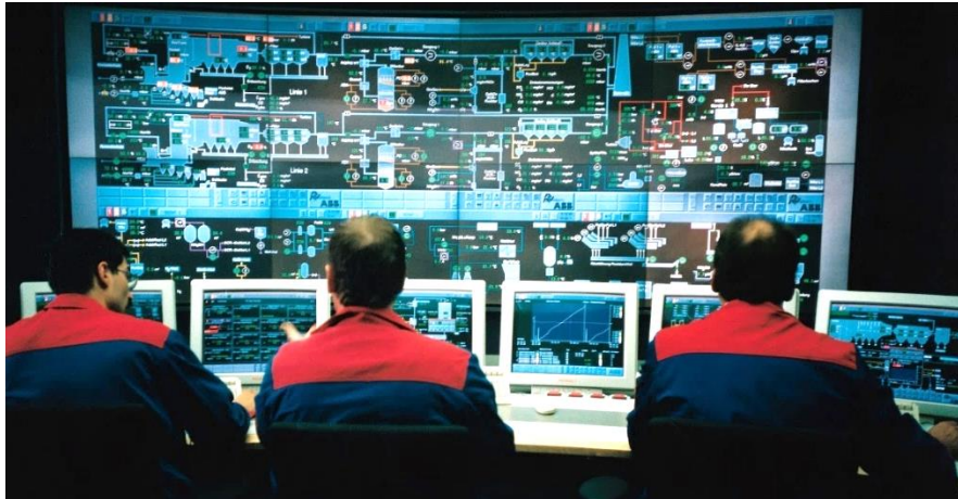
Figure 2 DCS Control Room
