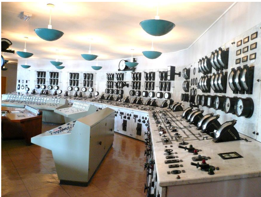
Figure 1 Pre-DCS/SCADA era Control Room
